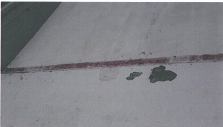
Spalled concrete at shallow end
