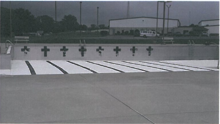
Peeling wall targets.
